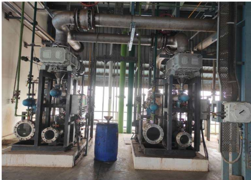
14. Reactor/Reaction Vessel, Condenser Vacuum Pump
